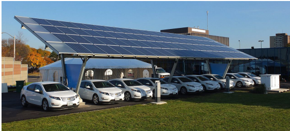
Figure: An EV Charging station
