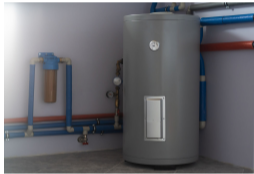
Electric water heaters
